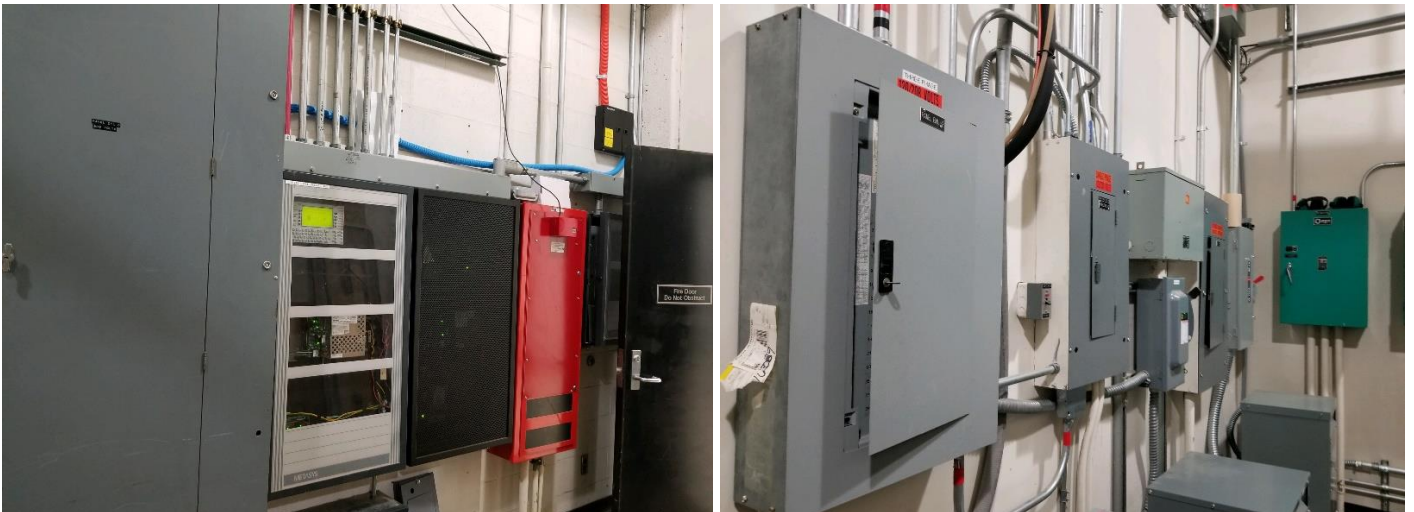
PHS – Building Automation Controls
